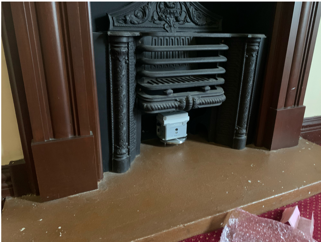
Figure 3: C22 Vibration Monitor (Kia Ora)
